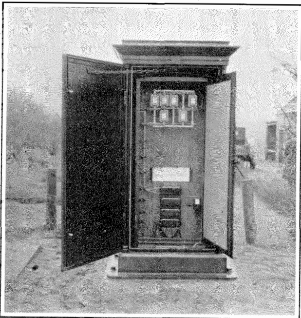
Figure 15—Interior of Cabinet—Transformer Side.
